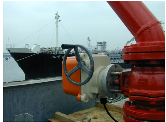
Chemistry pier, fire system
