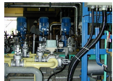
Power plant, fuel combustion system
