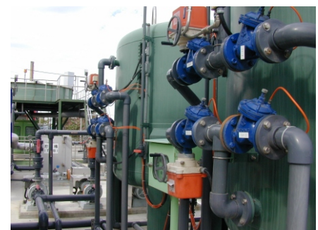
Oil-water separation treatment
