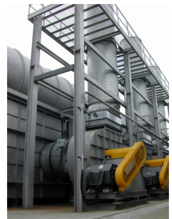
Damper control equipment
